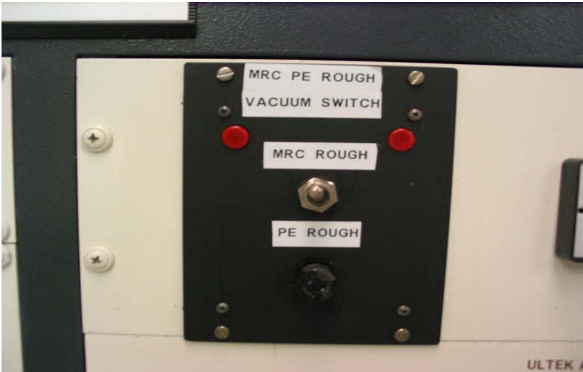
Figure 3 Rough Valve Switch
